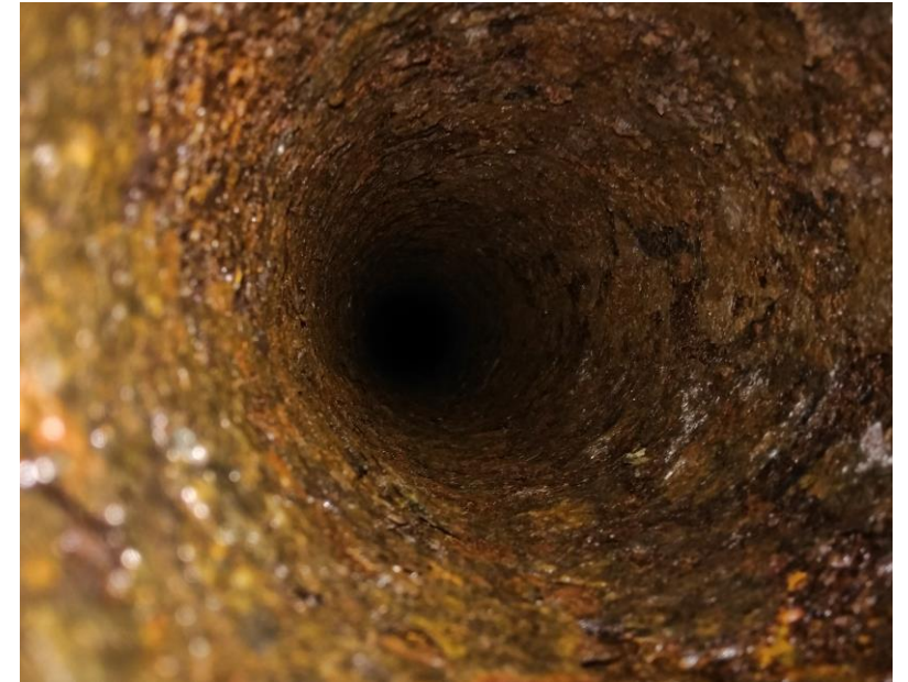
Rough walls of a corroded tube
